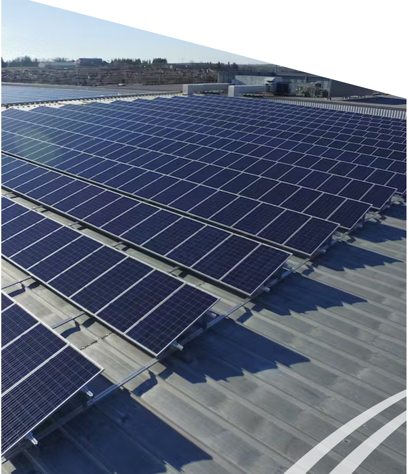
Solar panels, Newmarket. Photo by Town of Newmarket.
